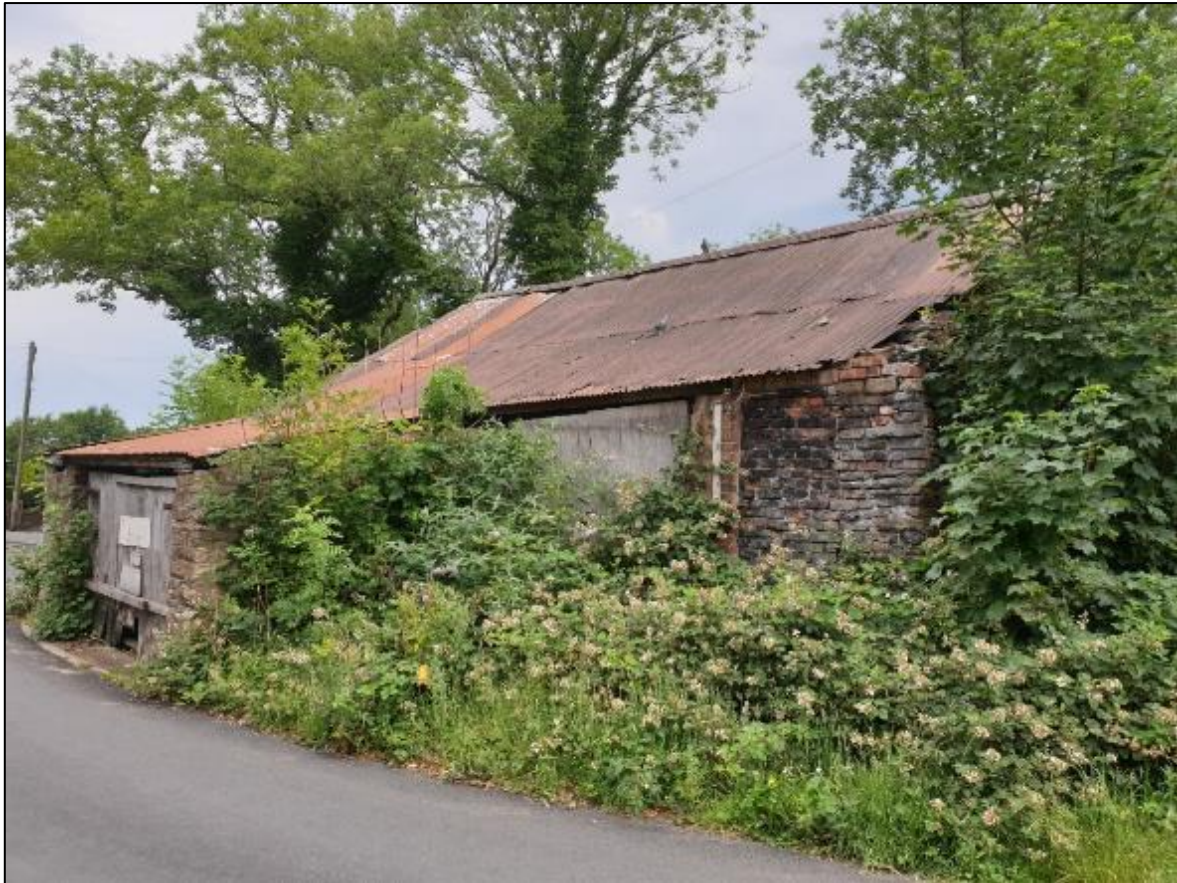
Plate 10 Outbuilding to the north of Apethorn Lane; although not within the Site, it is an integral part of the farmstead's development and is considered to be curtilage
