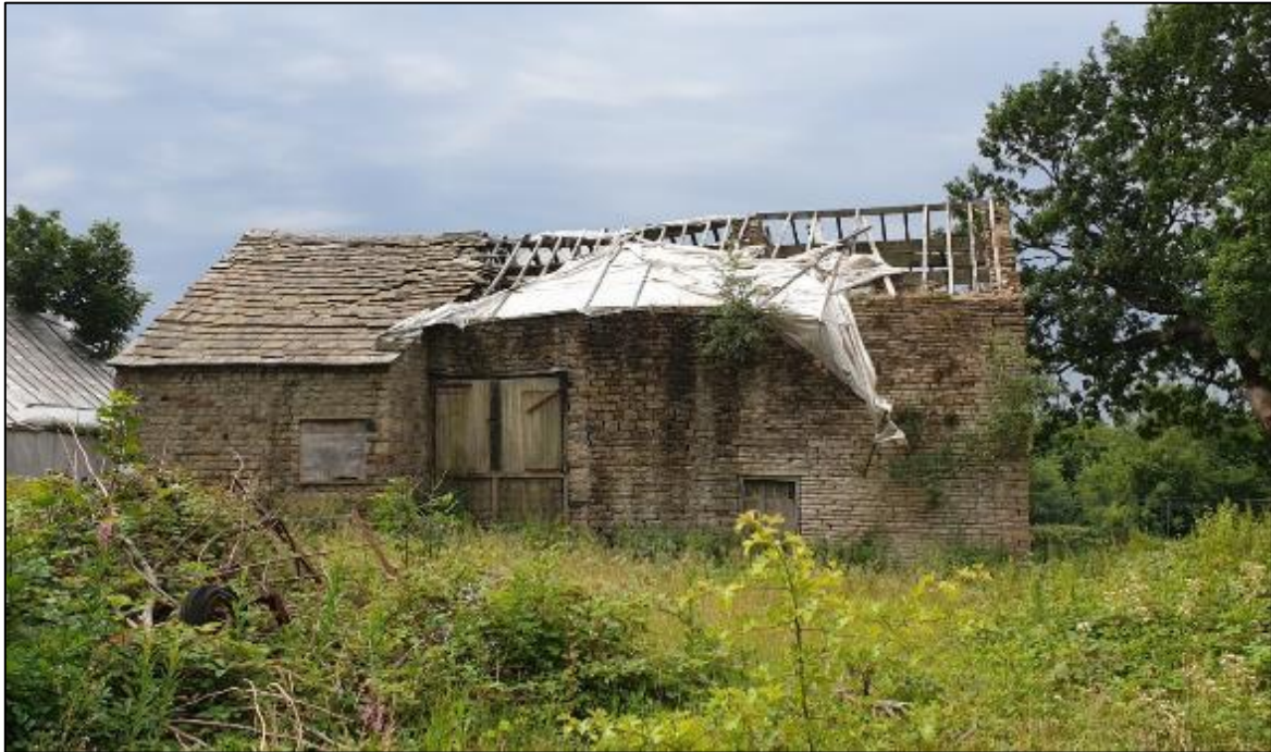
Plate 7 Combination Barn at Apethorn, probably mid-late 18th century. The left-hand side is the oldest part; the right-hand side was added in the mid-19th century
